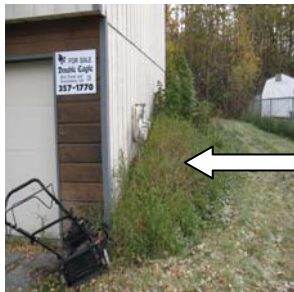
Vegetation encroaching on siding.
