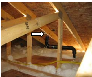
Bathroom vent duct dumps to attic.
