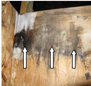
Mold on insulation bulkhead
