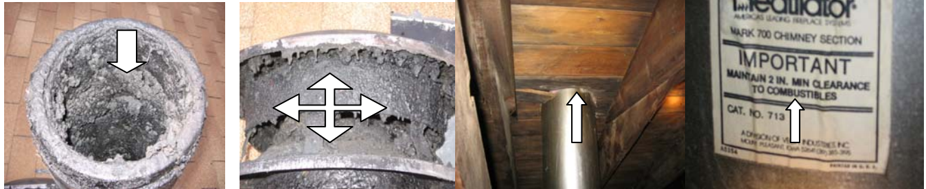
Creosote in wood stove stack.
