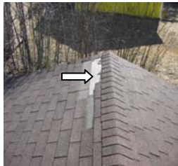
Shingles missing from roof
