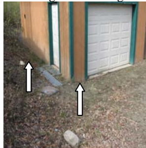
Siding soil contact.
