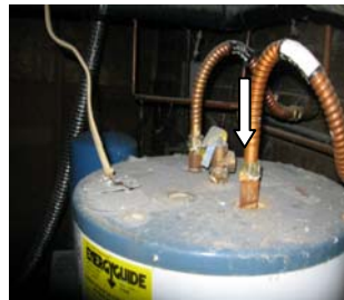
Missing PTRV extension
