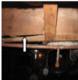
Cracked floor joist viewed from crawl space
