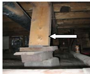
Floor joist support improperly installed.
