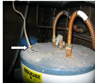
Protective bushing missing
